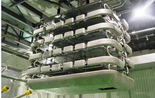
Fig. 3. The shielding covers for HVDC converter system
